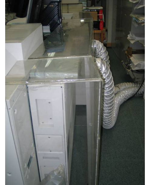
Dedicated Exhaust Duct for Digital Printer
