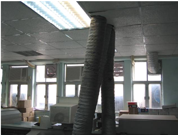
Dedicated Exhaust Ducts for Digital Printer
