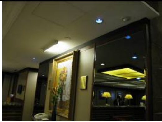
LED lights in lobby
