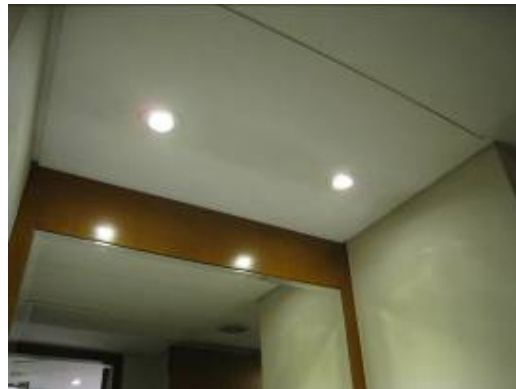
LED lights in guestroom
